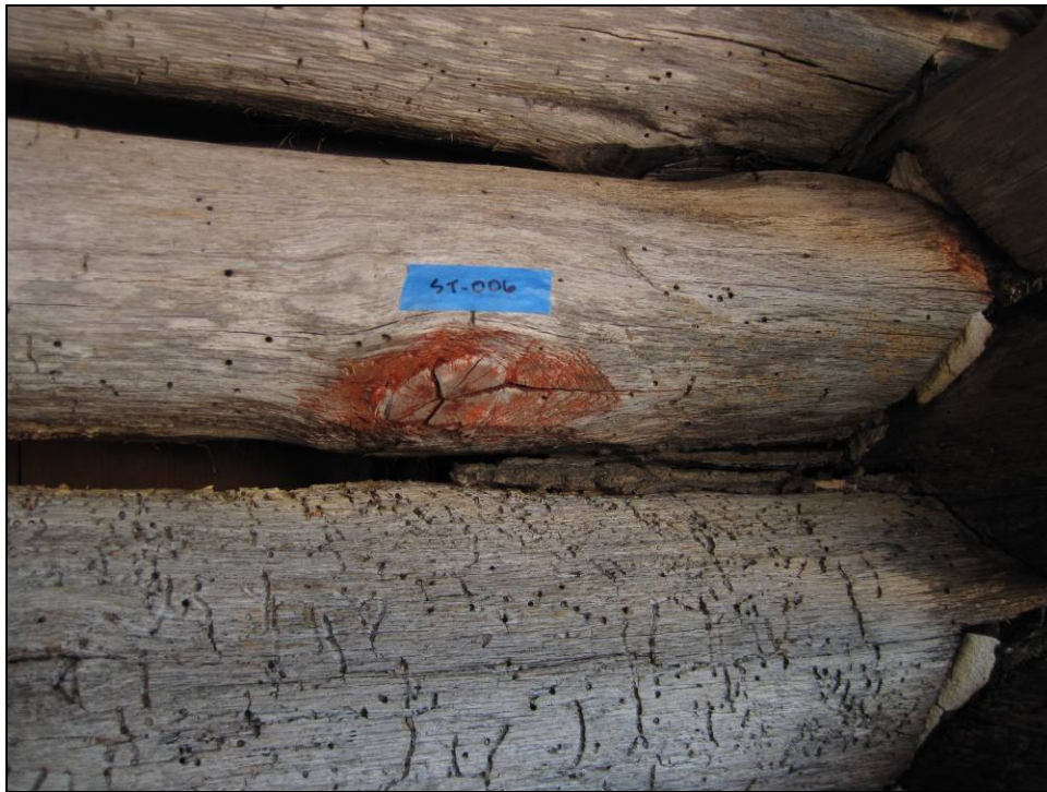
Figure 9: The chinking / daubing between the logs is mostly missing; where present, the chinking / daubing is severely deteriorated.
